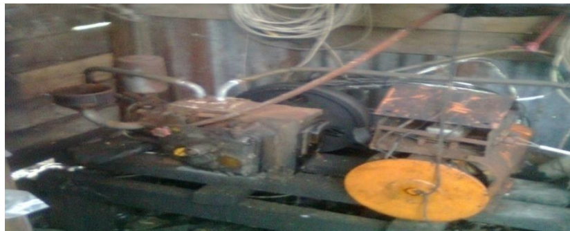
Gambar 13. Generator Set ( Genset )
